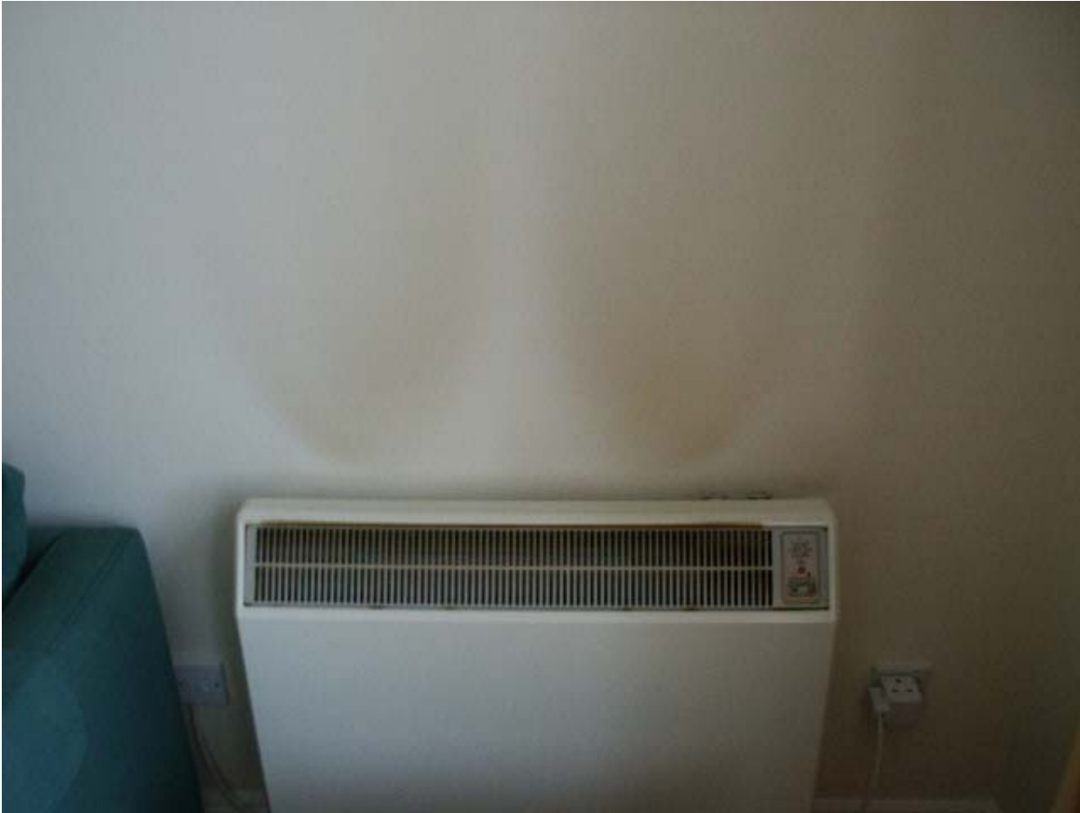
Reception Room – Heat marks above Dimplex heater.
