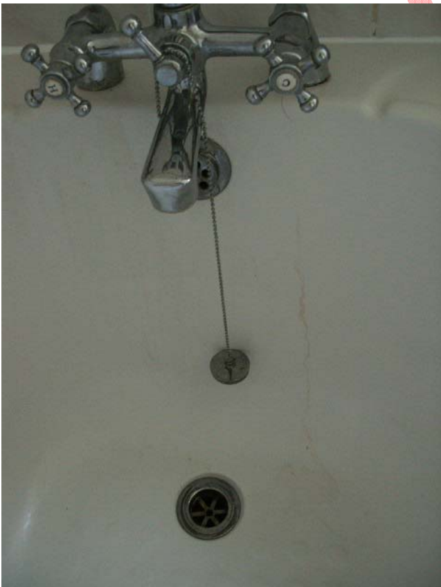
Bathroom – red drip mark
