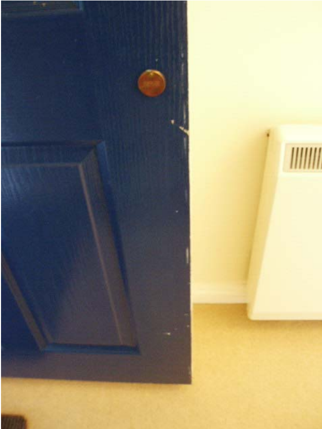
Entrance Hall – marks to entrance door
