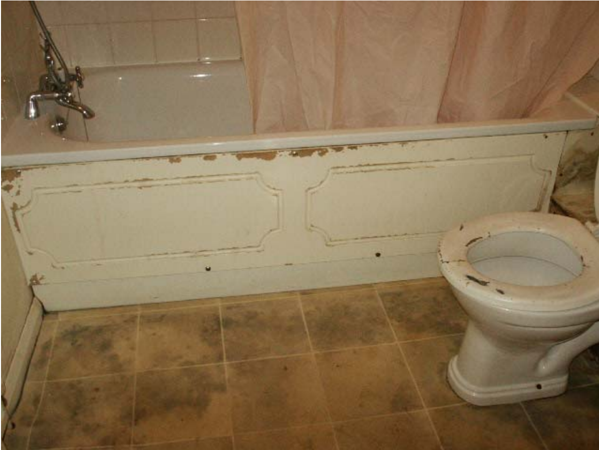
Bathroom – water damage to bath panel and floor
