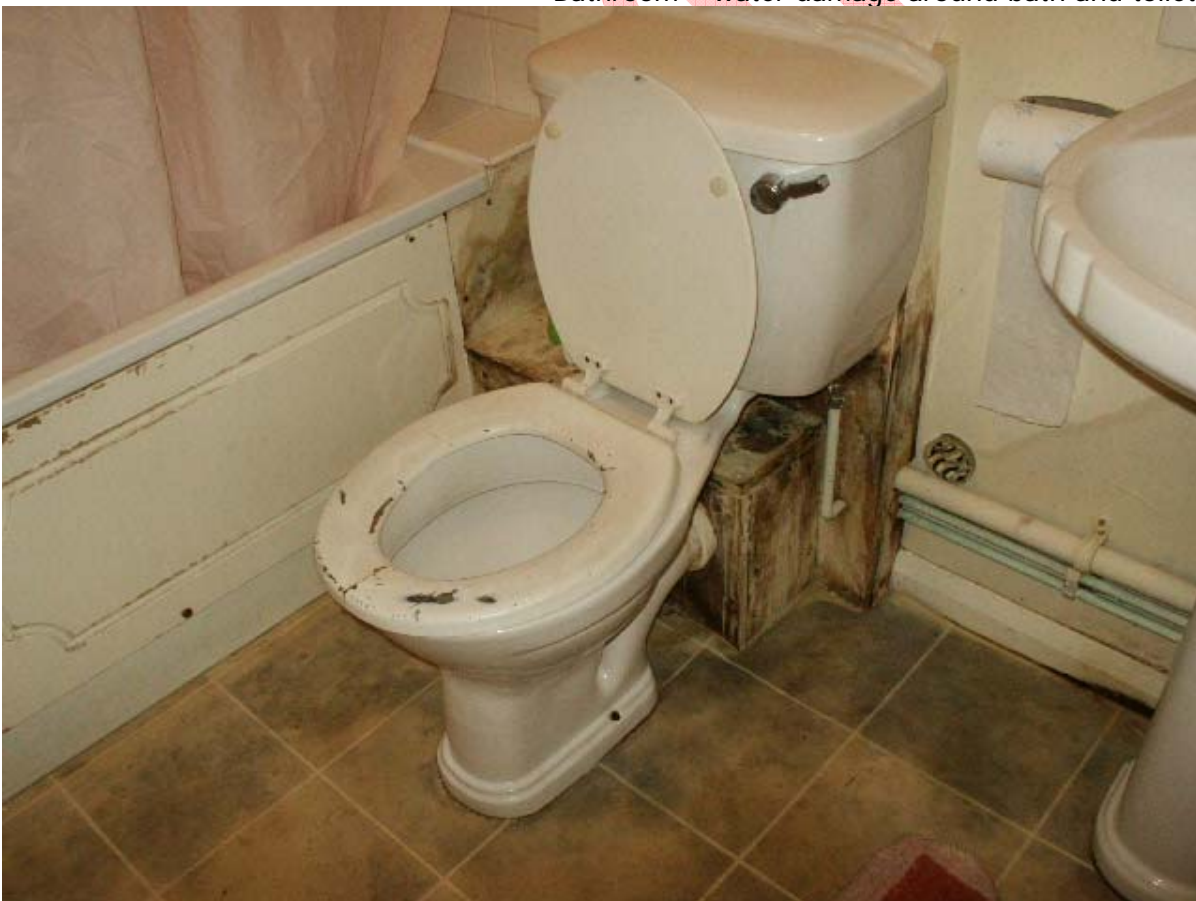
Bathroom – water damage around bath and toilet
